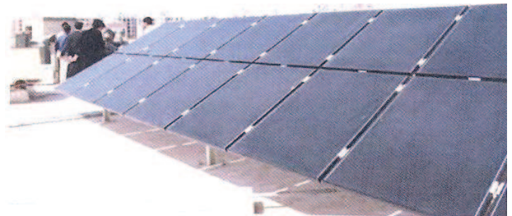
A view of one of the PV systems installed at NIT Gandhinagar.
